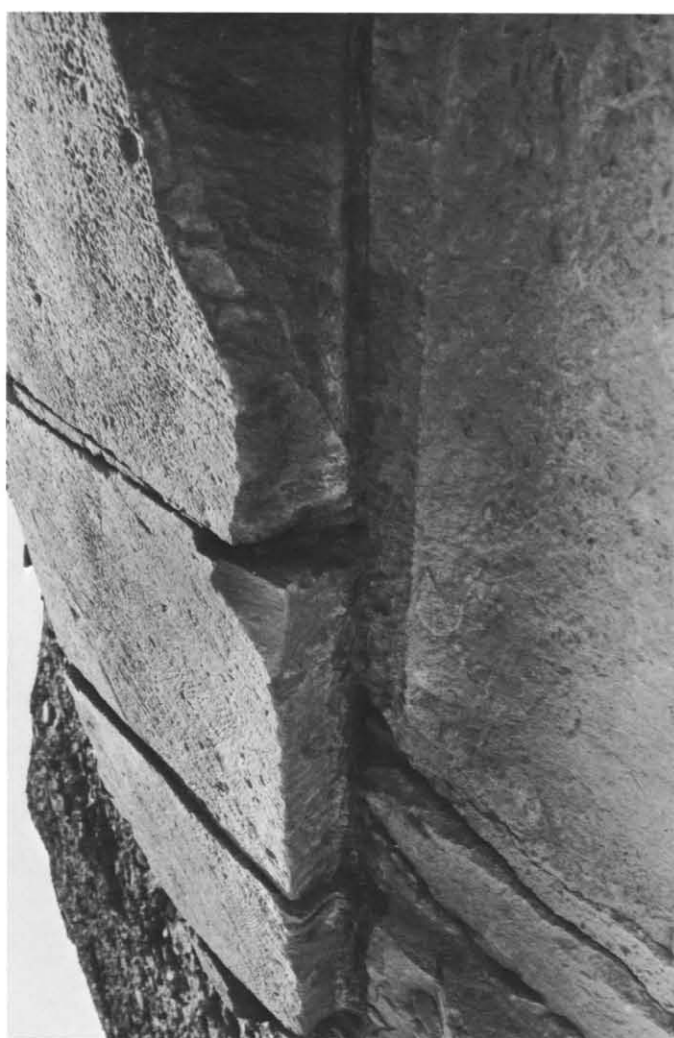
Pl. 41b: Cavity left by patching slabs of pyramid casing now fallen off.
