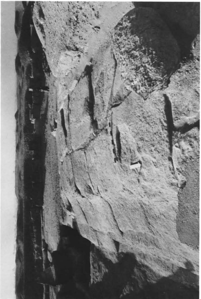
Pl. 39c: Remains of casing blocks at pyramid southeast corner. See pl. 95b.
