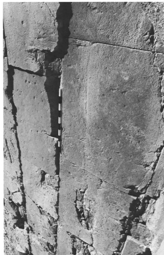
Pl. 40c: Course 5 of pyramid casing on west side of pyramid. See pl. 93a.
