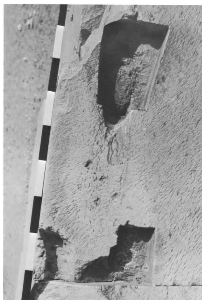
Pl. 5d: Dressed and repaired inner surface of Phase A wall of causeway.
