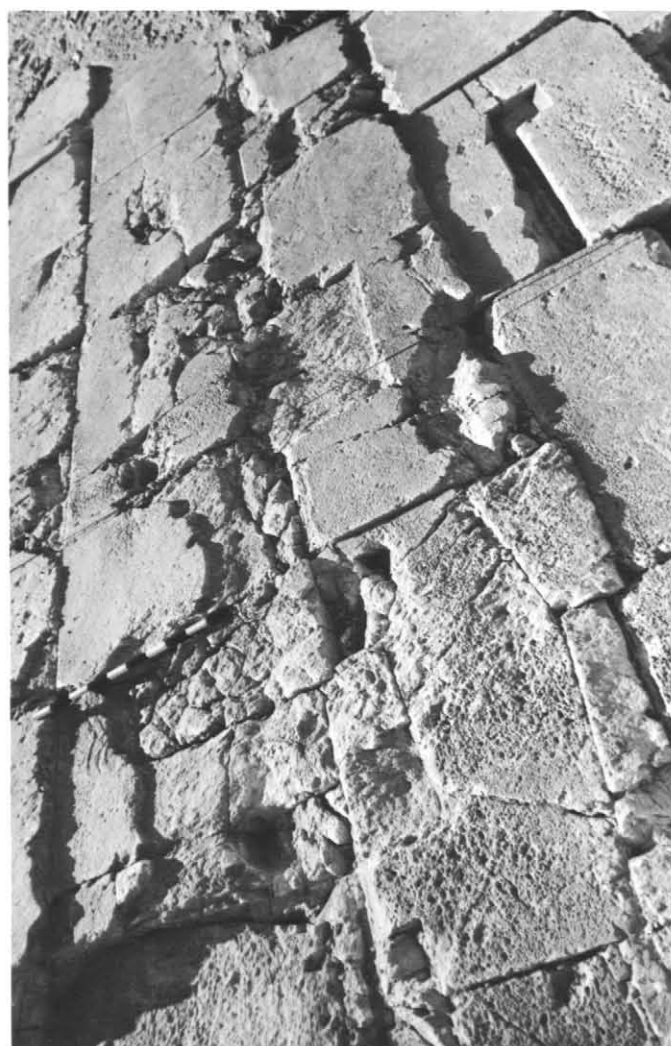
Pl. 40d: Damaged and repaired casing on west side of pyramid. See pl. 93a.
