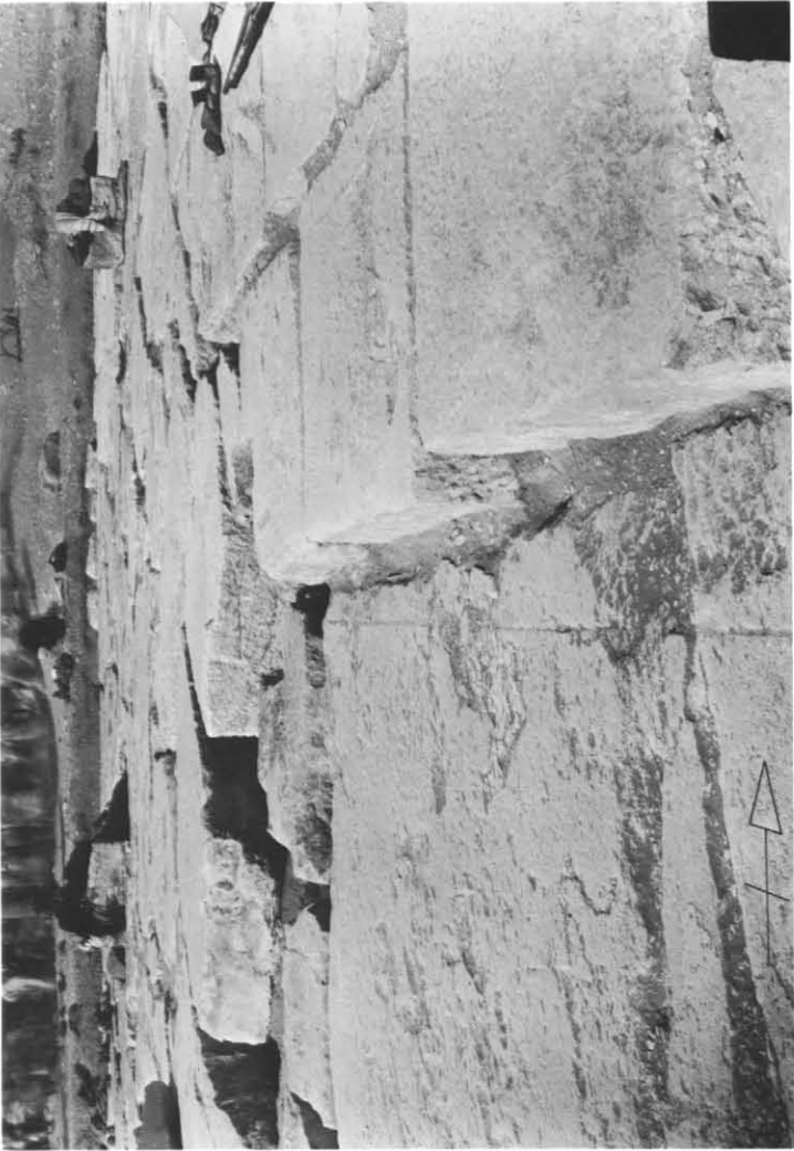
Pl. 29b: Foundations of northwest corner of pyramid and inner court. See pls. 87 and 94.
