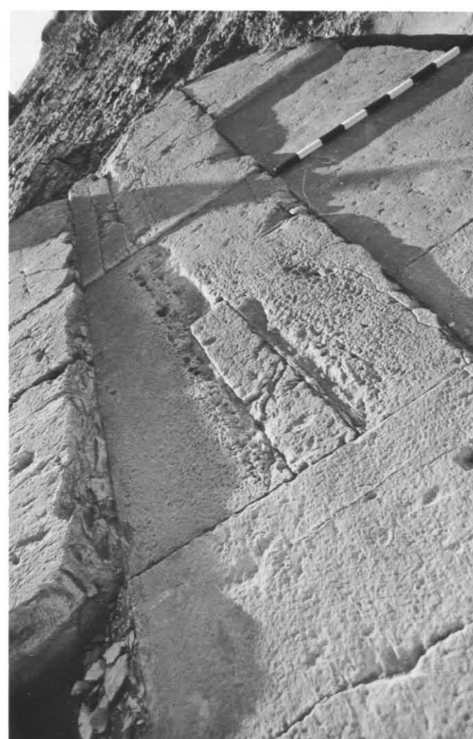
Pl. 41d: Repaired blocks in course 7 of pyramid west side. See pl. 93a.
