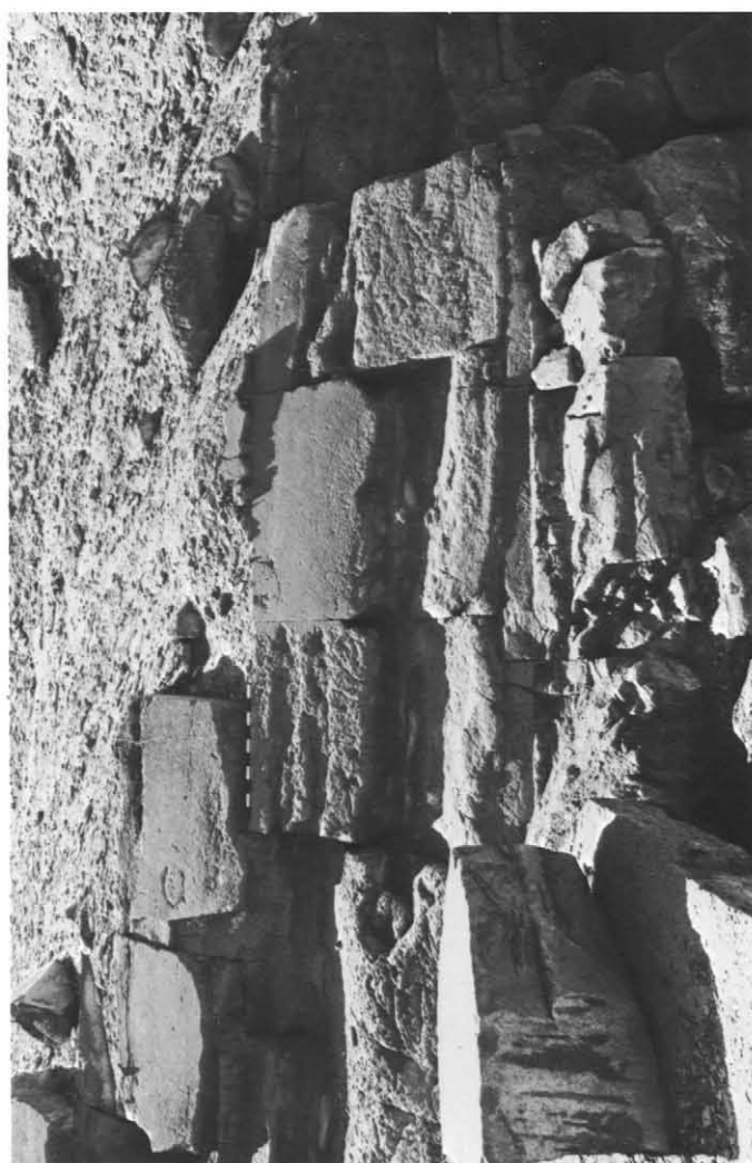
Pl. 40b: Damaged casing blocks east of pyramid entrance. See pl. 91.
